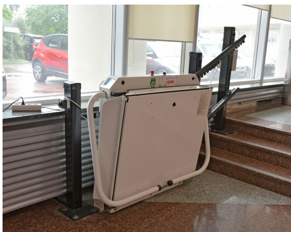
Architectural accessibility in Statistics Poland building. Platform for wheelchairs
