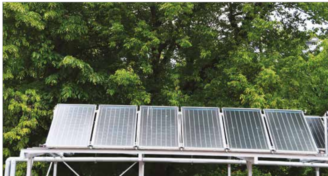
Photovoltaic panels at Statistics Poland building
